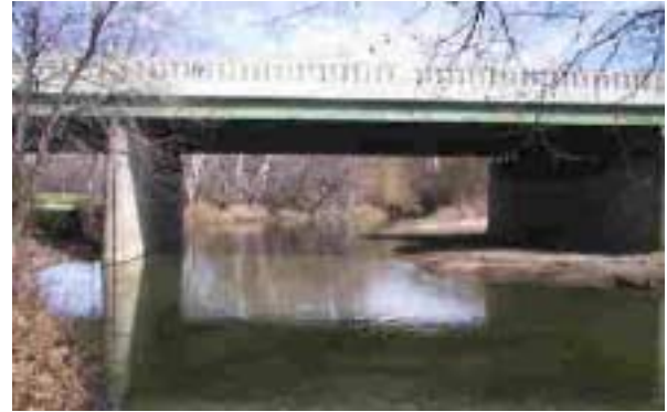
Figure 4. The Fall Creek at Millersville. The EasyQ is installed on the concrete bridge support.
